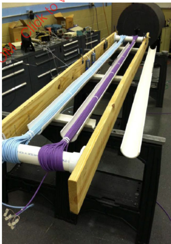
Figure 4 – Open conduit (Tray)
