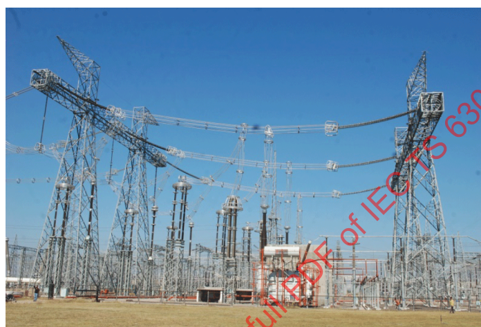
Figure B.13 – 1 200 kV national test station (India)
